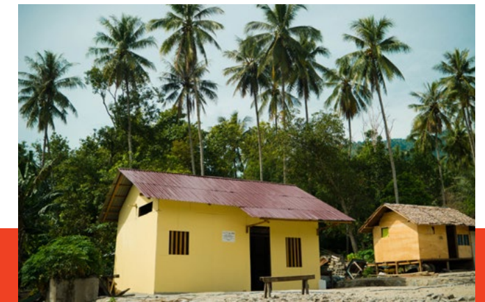
As the days after the disasters turned to months, we helped 220 families build transitional shelters, which are a more durable intermediate step as they prepare to rebuild permanent housing. Community members and local builders joined construction lessons in six villages.
